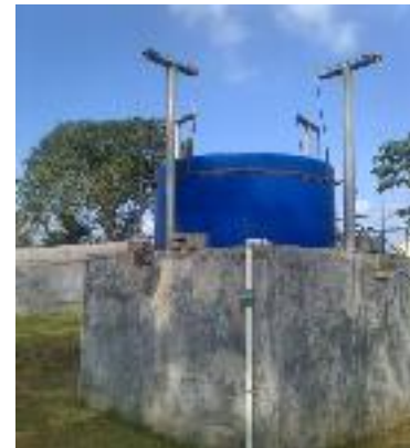
Figure 6. Biogas Holder tank (Blue collar)
