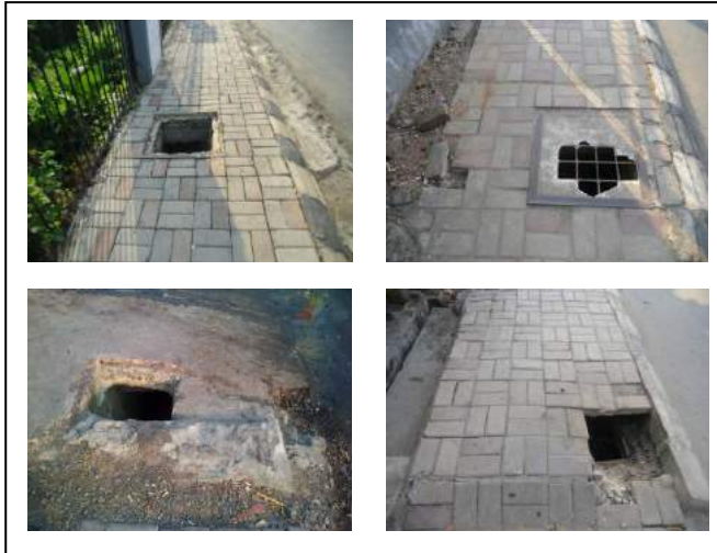
Figure 8. Drainage Hole Condition Source: Author
