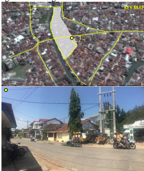
Figure 27. PLN electricity pole Kampong Jembatan Beton Way Blau [10]
