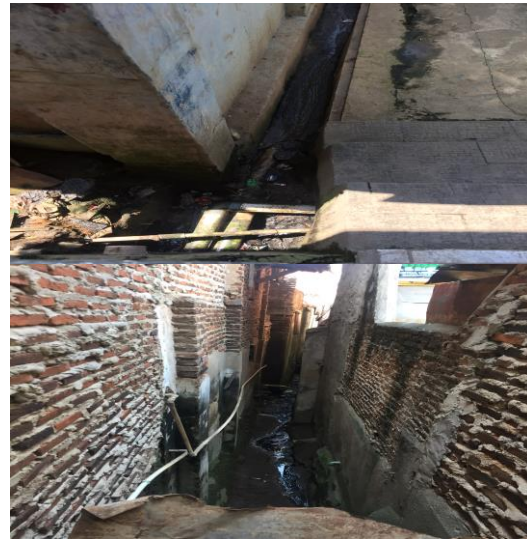
Figure 22. Drainage network Kampong Jembatan Beton Way Blau [10]
