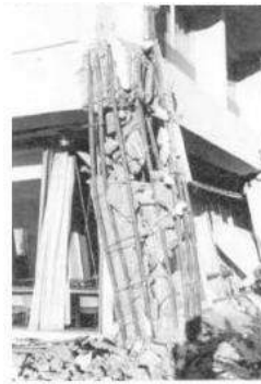
Fig. 11 The failure of reinforce concrete weak column Sources: Website Earthquakes and Earth's Layer
