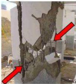
Fig. 9 Diagonal Cracks in Type of a Column Sources: Website Earthquakes and Earth's Layers
