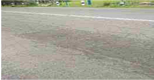
Gambar 2.15. Kerusakan Long and Trans Cracking
