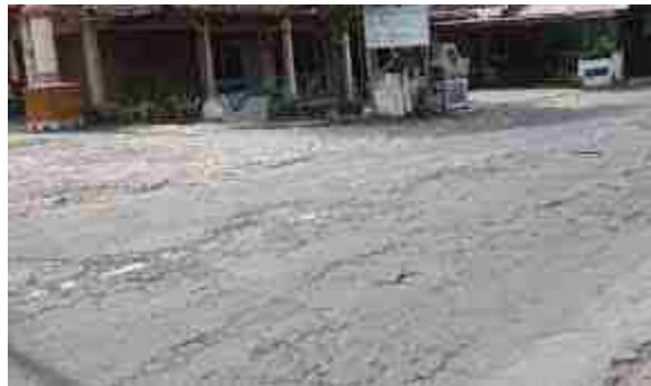
Gambar 2.13. Kerusakan Oil Spillage
