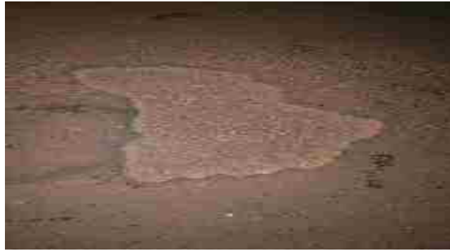
Gambar 2.6. Kerusakan Block Cracking
